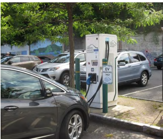
EV CHARGING STATION, BRATTLEBORO Photo Credit: WRC
