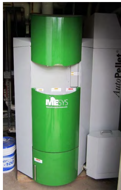
ADVANCED WOOD HEAT PELLET BOILER, MARLBORO ELEMENTARY SCHOOL Photo Credit: WRC
