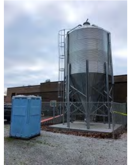
BULK PELLET STORAGE FOR ADVANCED HEAT SYSTEM, DUMMERSTON ELEMENTARY Photo Credit: WRC
