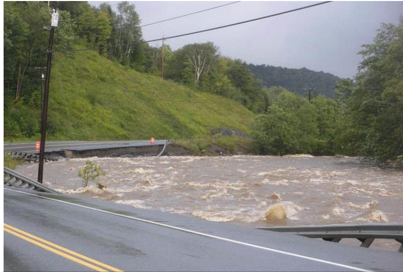
This photo shows the real connection of river and road during TS Irene, as the river reclaims its floodplain, edging in on the road. Photo courtesy of wilmingtonvtfloodingrelief.com .
