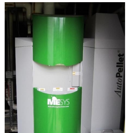
ADVANCED WOOD HEAT PELLET BOILER, MARLBORO ELEMENTARY SCHOOL Photo Credit: WRC
