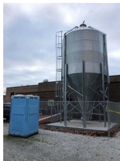
BULK PELLET STORAGE FOR ADVANCED HEAT SYSTEM, DUMMERSTON ELEMENTARY Photo Credit: WRC
