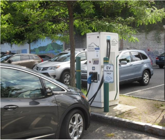
EV CHARGING STATION, BRATTLEBORO Photo Credit: WRC
