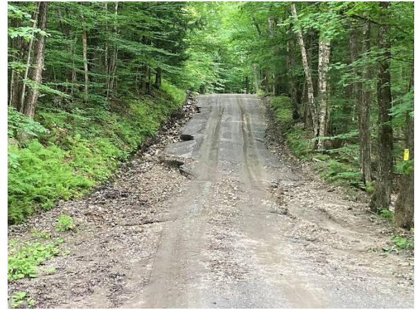
DAMAGE TO BACK WINDHAM ROAD, TOWNSHEND, JULY 2021 Photo Credit: WRC
