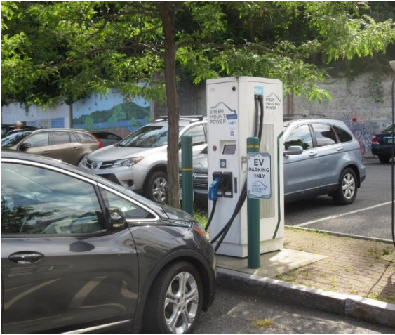
EV CHARGING STATION, BRATTLEBORO Photo Credit: WRC
